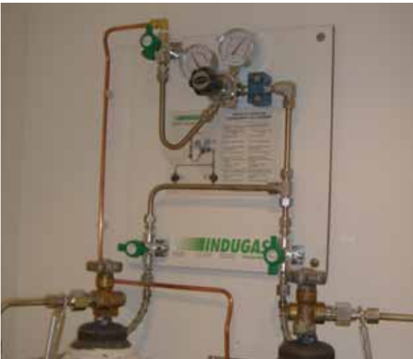
Fig. 3. — Central oxygen distribution
